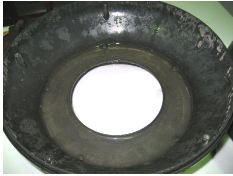
Figure 6 – Sample 2, water pooling inside housing and dripping down inside of enclosure
