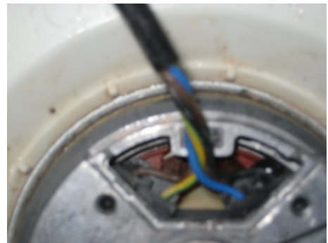
Figure 4 – Sample 1, minimal water on fan motor housing and no water inside fan motor
